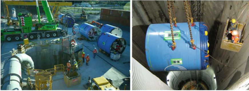
Fig. 2.4 Tunnel access shaft and TBM components/TBM segment being lowered for assembly below ground
