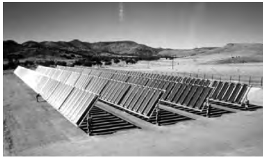
Fig. 1.9. A two-axis tracking 100-kW ENTECH power plant in Texas. System efficiency of up to 14% was demonstrated with this technology at 20 suns: curved Fresnel lenses showed optical efficiency of over 85%. Different cells were used to make the receivers
